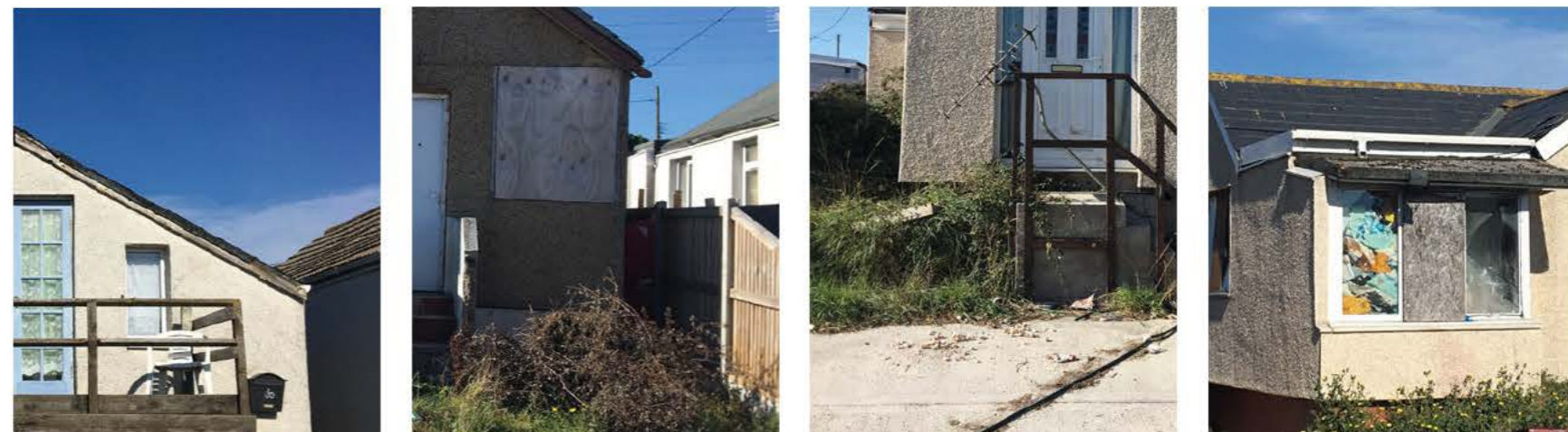
Fig. 49. Examples of occupied housing in poor condition.
