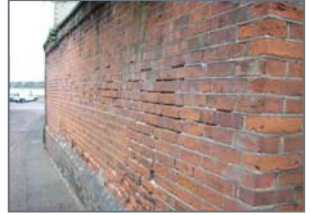
Important brick wall forming curtilage of Listed Building where pointing has failed
