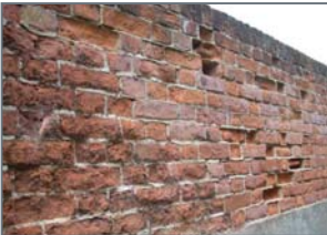
Heavily eroded soft red brick wall in need of extensive repair
