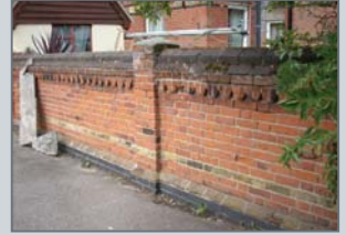
Boundary wall in Harwich with a mix of brick types and colours
