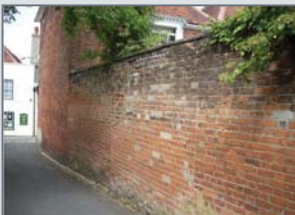
Unattractive cement patch repairs on important historic wall forming curtilage to a Listed Building
