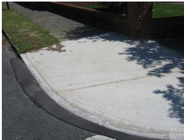
Public realm: A manual would promote better materials and detailing than this highly visible mass concrete street corner.
