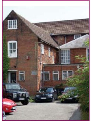
Single, two and three storey rear extensions of varying form and quality
