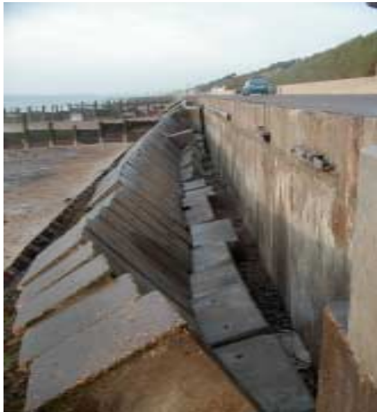
Failed sea wall at Holland
