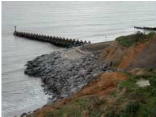
Rock armour Work at the Naze to prevent outflanking of the sea wall
